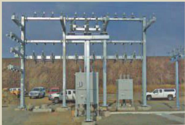
Pilotec Substation Location: Mountain Iron, MN Date Galvanized: 2008 Project Maintenance: 72 years
